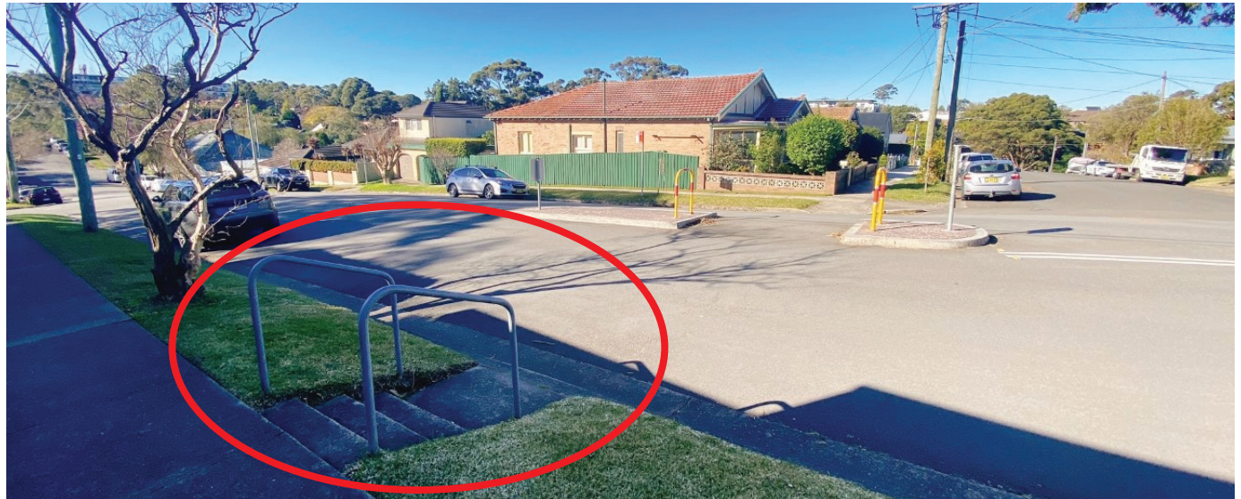
Pedestrian crossing without a ramp (south of Cobar St)
