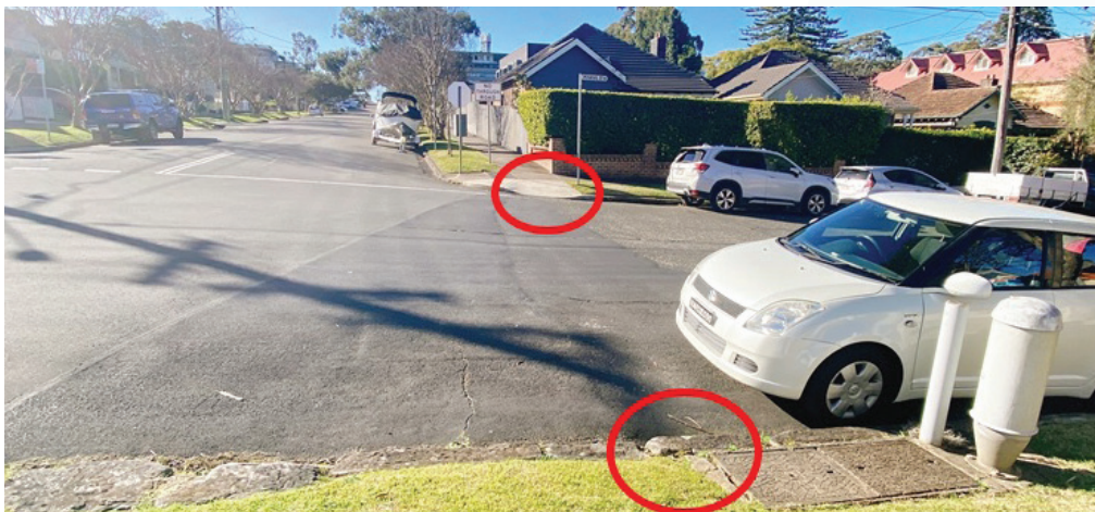
Missing pedestrian ramp on Penkivil Street and Penshurst Street intersection
